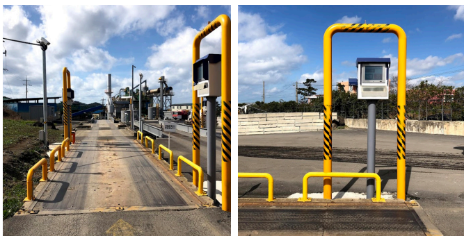
Weighbridge and automatic measuring equipment installed at the entrance of a waste disposal facility
