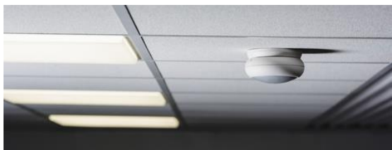
Security, environment control
