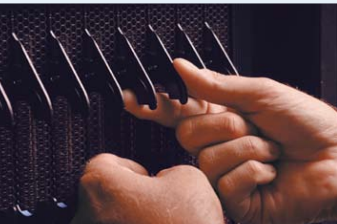
Left: Blade servers at an Intel data center
